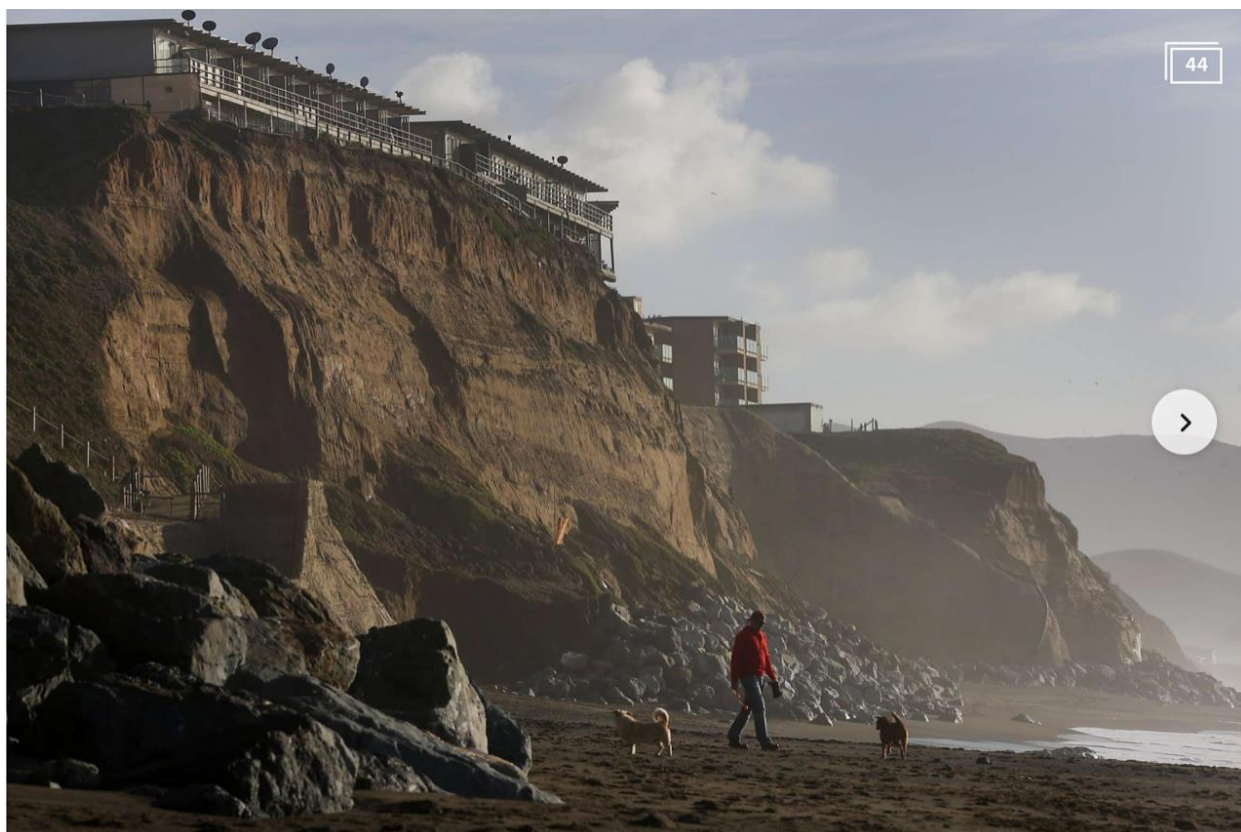
Properties along Esplanade Ave can be seen perched on the edge of an eroding cliff Dec. 23, 2015, in Pacifica, Calif. The center property is vacant. (Leah Millis/San Francisco Chronicle)
